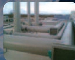
External Ducting Systems and fans
